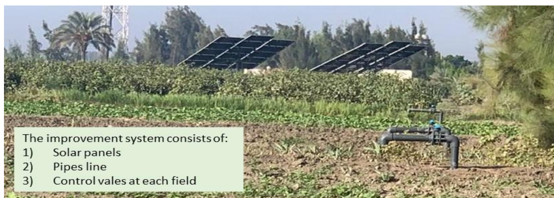
Figure 16. The Solar powered irrigation system: Solar panels – Pipe system – control valves.
